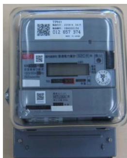
Photo 7-1 KEPC smart meter
